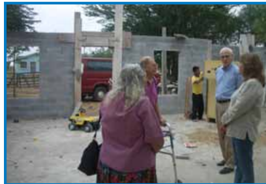
Pedro and Maria Rodriguez share the progress on their home with CRG staff.
